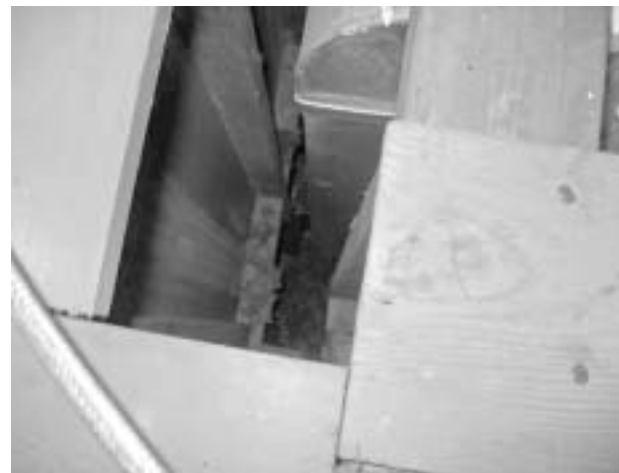
This large opening let attic air into the living space, wasting energy.
